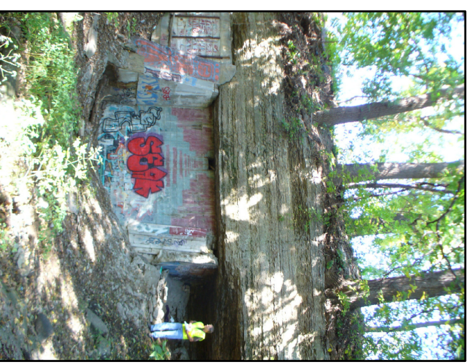
Discharge Location Cross Sections St. Anthony Falls East Bank Restoration St. Anthony Falls, Minneapolis, Minnesota
